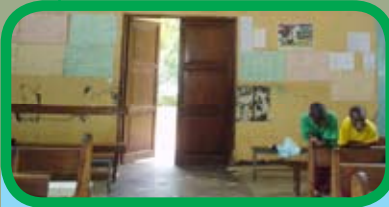
Peeled off PVC Tiles along the Isle from Entrance Porch towards the Pulpit
