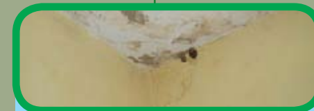
Cracked wall and slab in the Chaplain's office. These sections with structural cracks shall require reconstruction.
