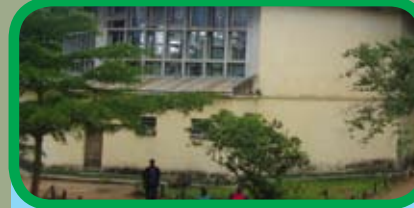
Gci sheets covering the Concrete Roofs slabs over Chaplain's office, Prayer cubicle and Entrance porch.
