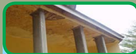
Spalling Concrete Slab over Entrance porch. Presently covered with cgi sheets
