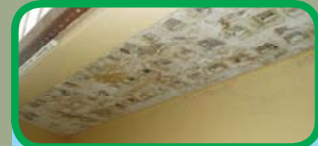
Leakages in the Roof over Prayer cubicle resulting from moisture ingress into the slab but no major structural crack observed
